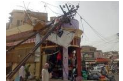
Damaged electric pole in Rajasthan, India. Credit: Reuters
