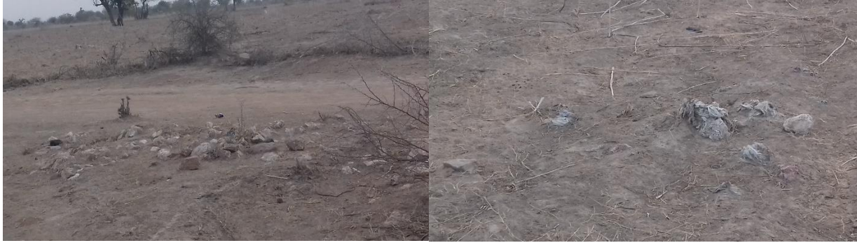
Stone bunds and remnants of sand bags used for erosion control in Kofa CDA (Katsina State).
