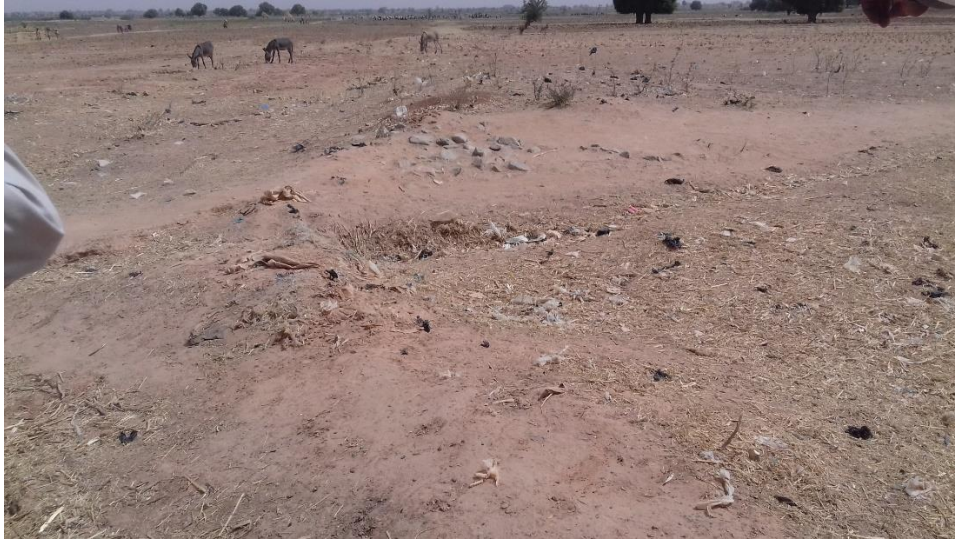
Bunds made of stones and sand bags to control runoff in Goran CDA (Zamfara State).
