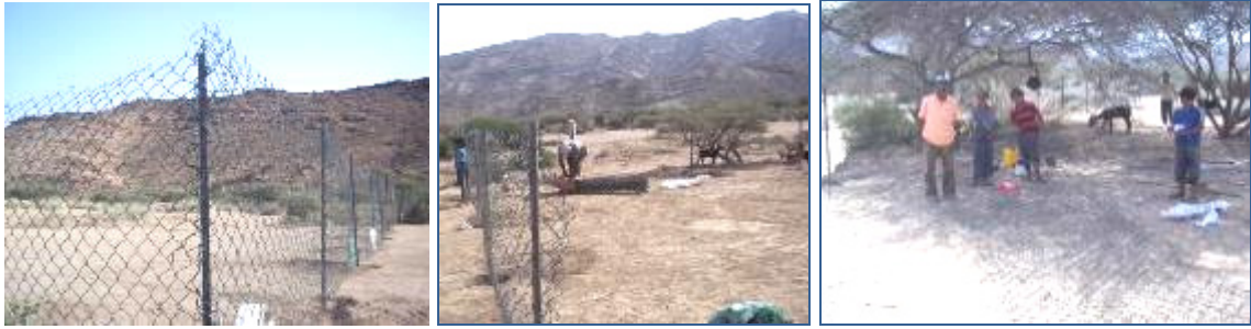
Figure 12. Some of the construction activities for an enclosed area at a pilot site in Yemen
