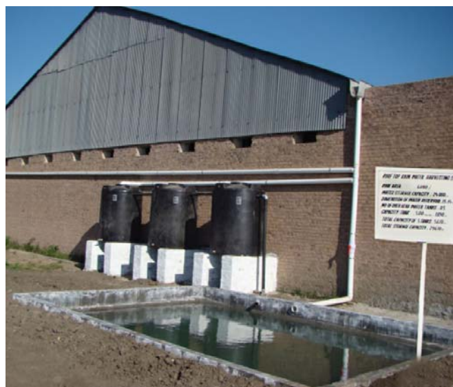
A rooftop rainwater harvesting system coupled with low pressure drip irrigation system in Chakwal, Pakistan.
