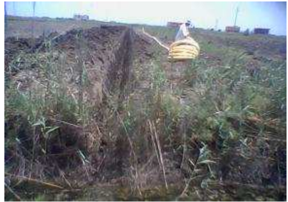
PVC pipes in location
