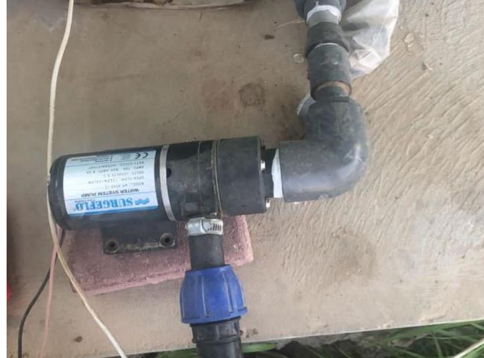
12V, 0.2 HP pump, powered by solar energy
