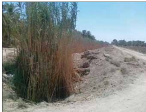
Figure 26. Surface drain in Mussaiab overgrown with weeds.
