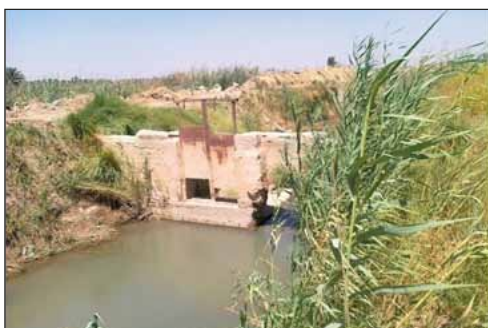
Figure 24. A main canal in the Mussaiab Irrigation Project showing loss of canal shape and poor condition of regulator.
