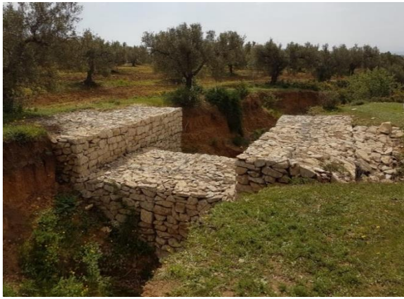
Figure 24: Gabion threshold installed on the wadi bed in Sbahia, (Zaghouan) to protect the land against the lateral landslides and improve olive production. Field photo, 23/03/2017.
