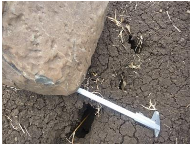
Figure 30: Cracks in the soil at the beginning of the rainy season
