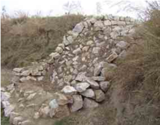
Figure 5.22. Stone spillway to divert excessive rainfall in a non-erosive way
