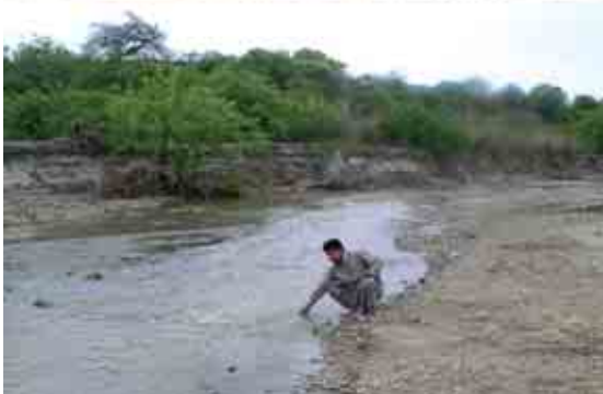
Stream bank cutting and gravity erosion
