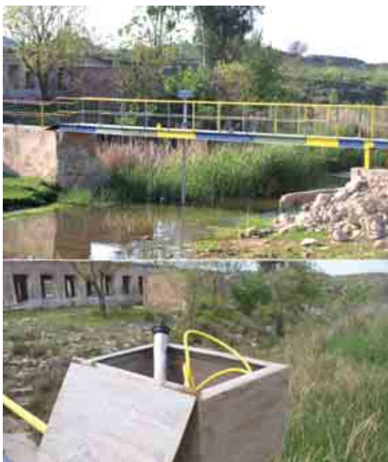
Water-level recorder installed at Chak Khushi
