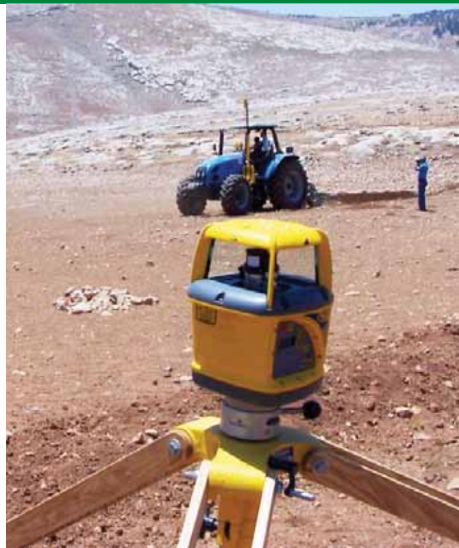
Laser guiding GPS-based system that allows the Vallerani unit to excavate contour lines without costly topographic work
