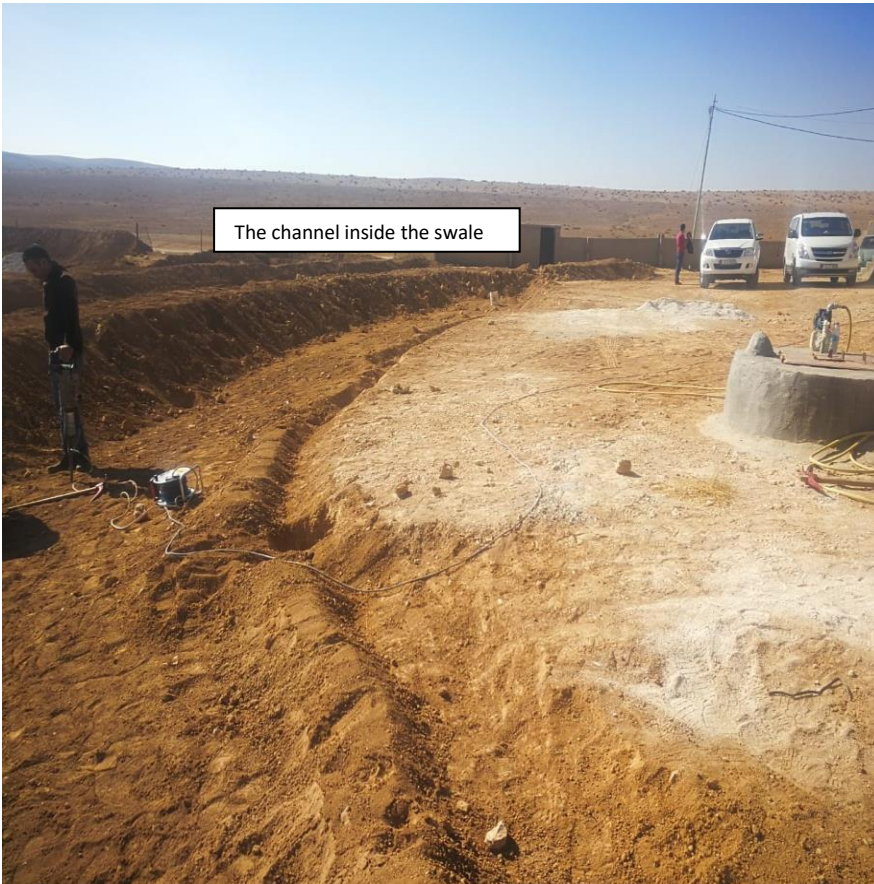
4) Digging holes inside the Canal that was previously designed to plant trees
