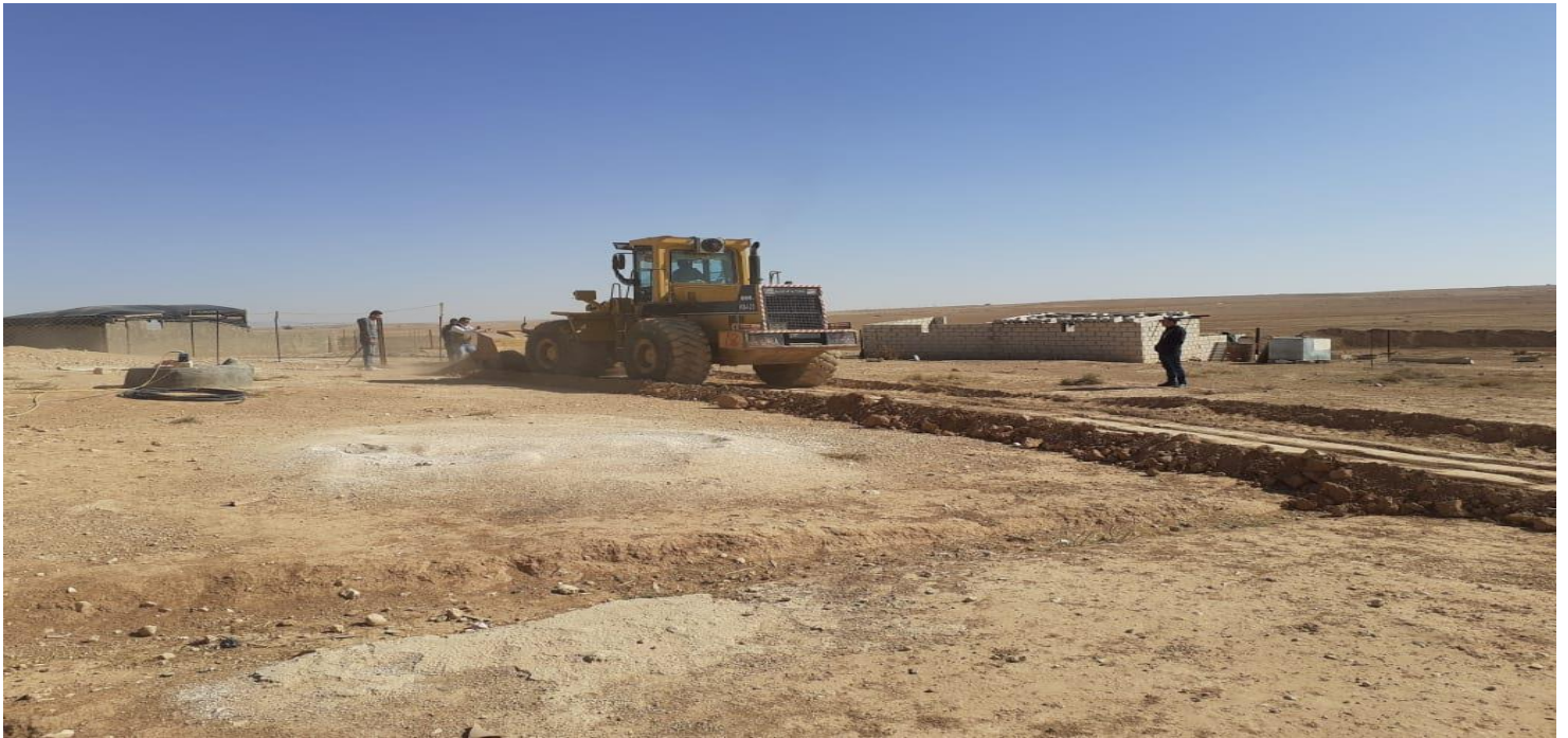
2- Digging the interior part of the Swale and put the soil resulted up the lower end of the Swale
