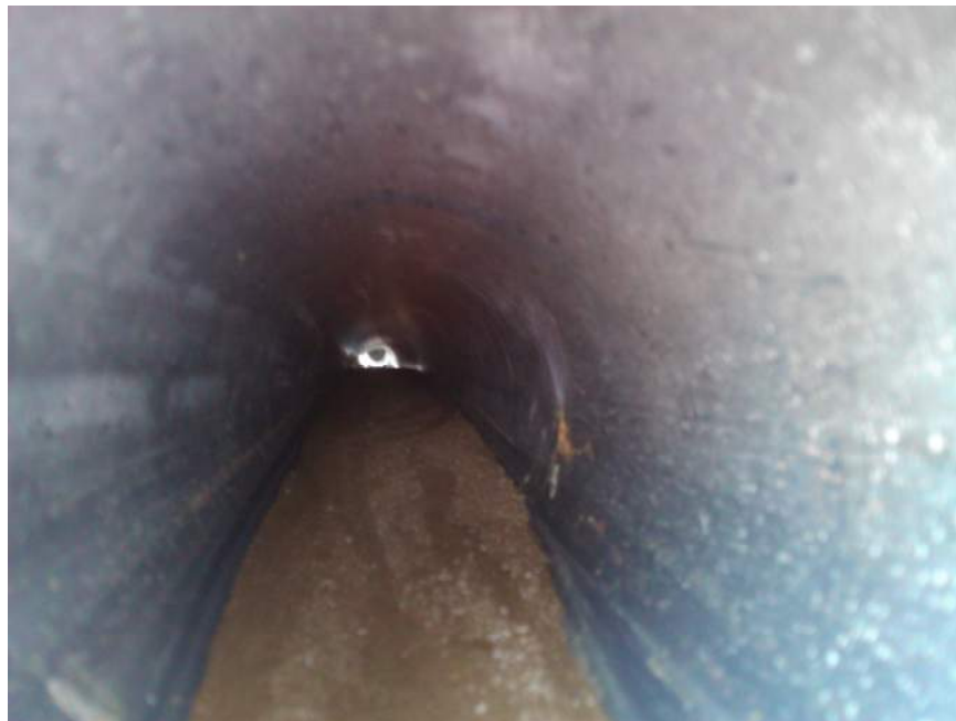
Figure 37: Clogged tube of the untreated plot
