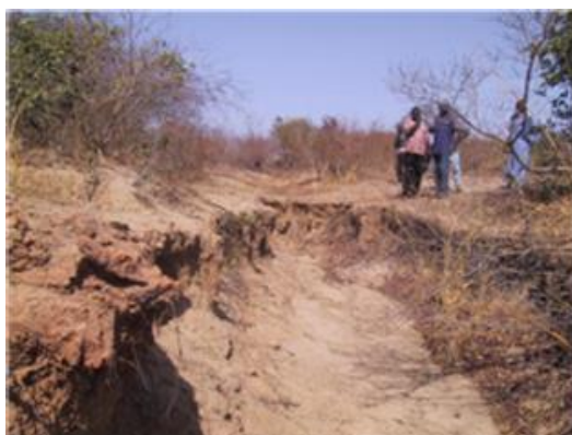
Water erosion (photo: JICA)
