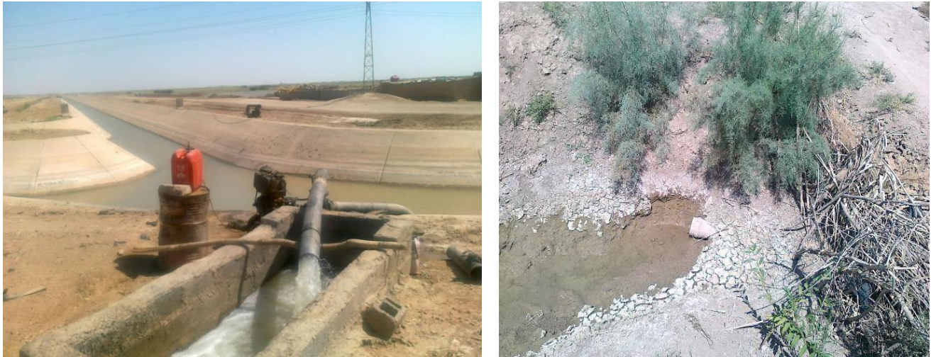
Figure 8: Illegal pump installed on irrigation canals and view of a choked drain.
