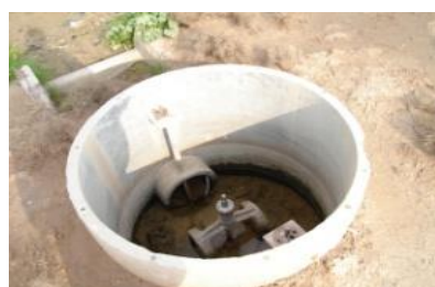
Figure 6: View of collector drain, damaged bridge and electromechanical regulators.
